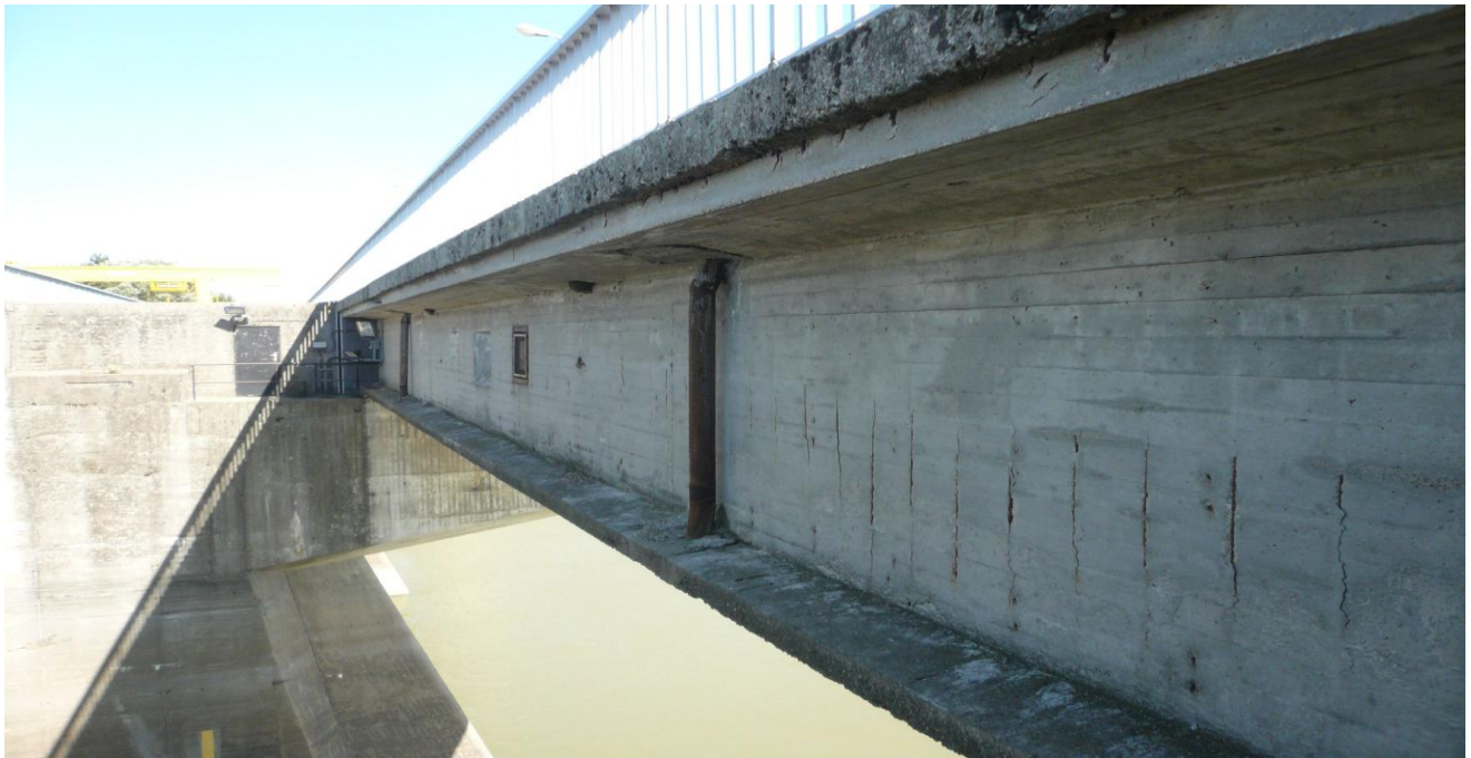
Figure 5 Cracks Along the Side Wall of Bridge
